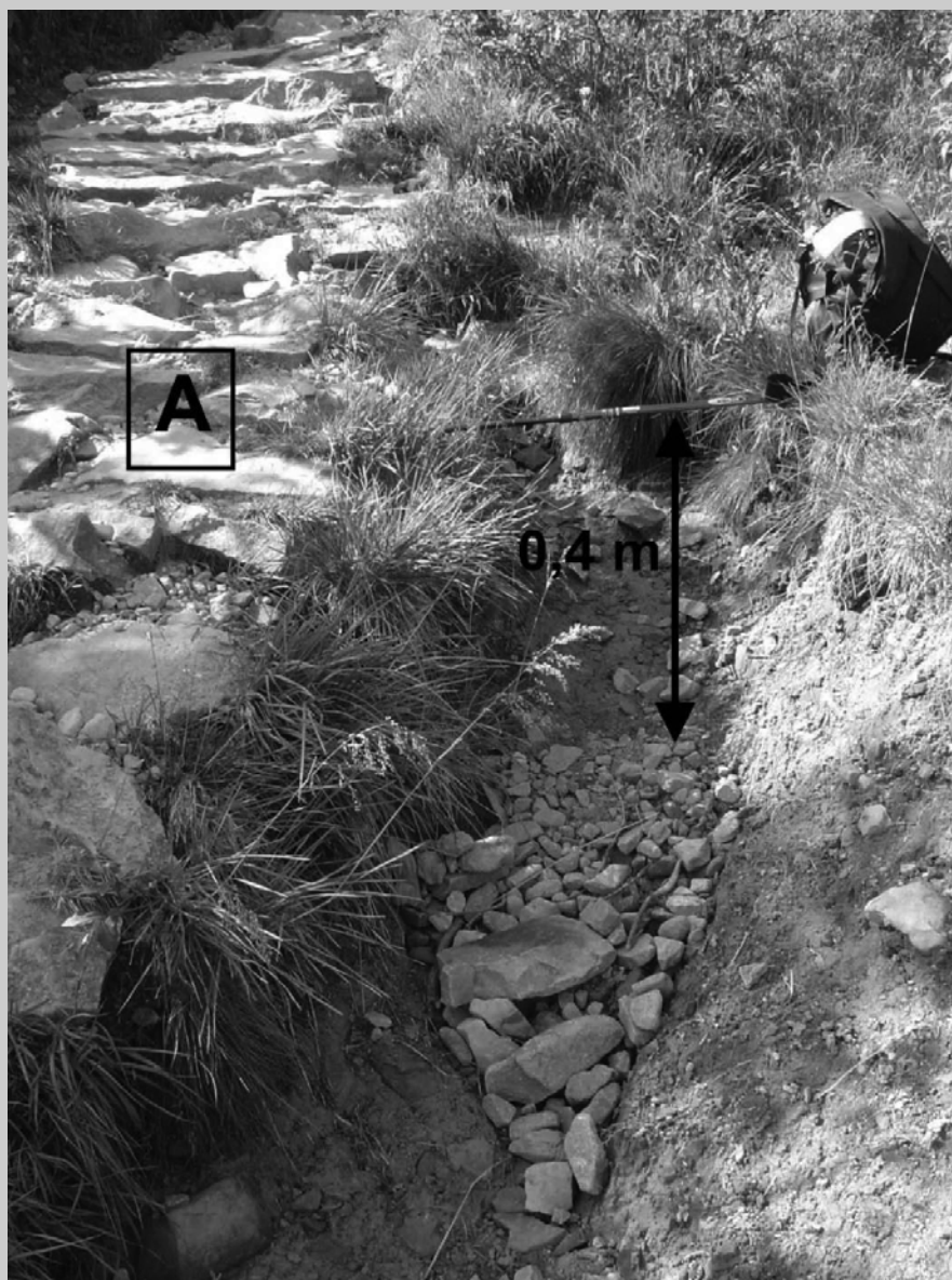
Fig. 10 An erosive cut along the trail near the Brona Pass (1408 m a. s. l.) in the Babia Góra massif with the maximum incision of 0.4 m. A boulder surface of the footpath (A) seems to be the most resistant to erosion induced both by natural and anthropogenic factors
